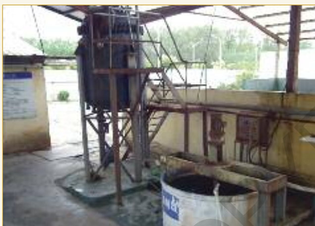
Chrome regeneration and reuse is practised. After precipitation and dewatering the chrome precipitate to 40% moisture, the chromium hydroxide is dissolved in sulfuric acid in the mixing vessel. The solution is then pumped to the elevated reactor vessel where it is steam heated, then chemically treated to remove residual protein from the complex.
