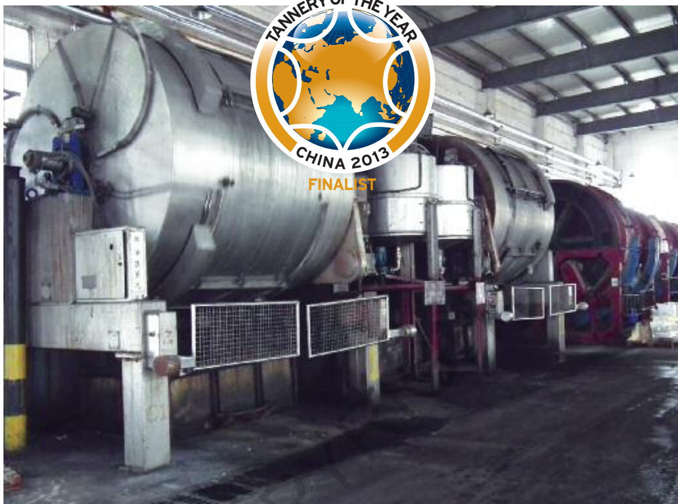
The dyeing department comprises a mixture of seventeen wooden and tri-compartmental vessels. The two vessels shown are of Chinese manufacture, are newly installed, and process loads of 2.5 tonnes shaved weight respectively.
