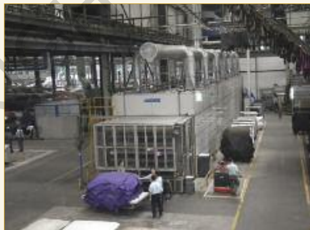
After samm setting and wet stretching, sides are loaded into the TAIC drying and conditioning unit. The leathers are held flat and conveyed forward with return several times at different levels to utilise the internal volume to its full capacity, before vibration staking.
