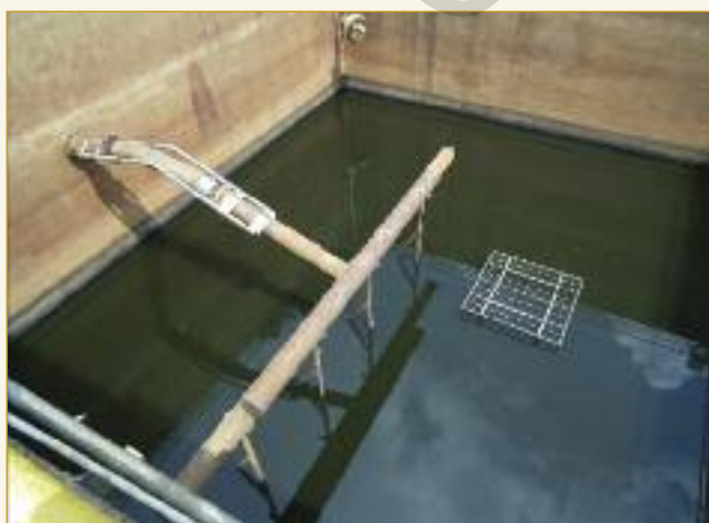
This picture shows the air inlet system in one of PrimeAsia China's submerged bio reactors, which forms part of the tannery's extensive effluent treatment system.
