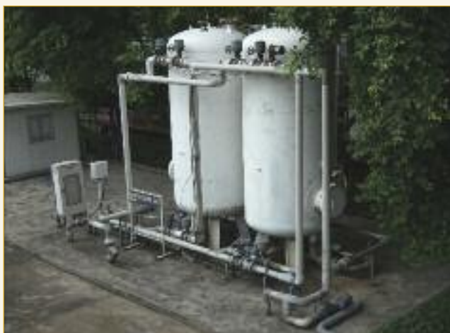
All of the treated effluent receives filtration through activated carbon columns to remove residual colour. Approximately 50% of this water is reused within the plant, the balance discharged as treated effluent.
