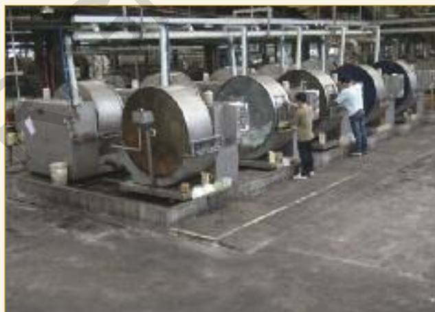
This section of the pilot plant comprised 10 stainless steel drums. In an adjacent area drums of various sizes are fitted to enable production of batches from single pieces up to 40 sides.
