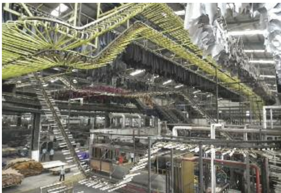
Drying conveyors are used extensively throughout the tannery. These systems are complex, and are only fully appreciated when they are not fully loaded with sides.
