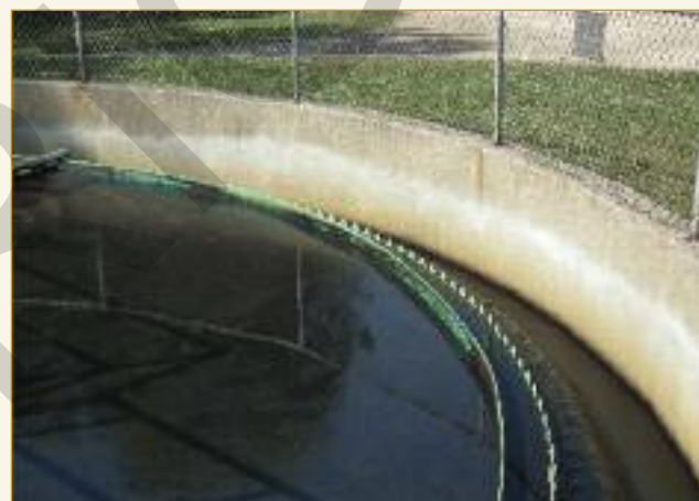
Primary clarifiers operate in parallel for settling of suspended solids after screening to remove gross solids.
