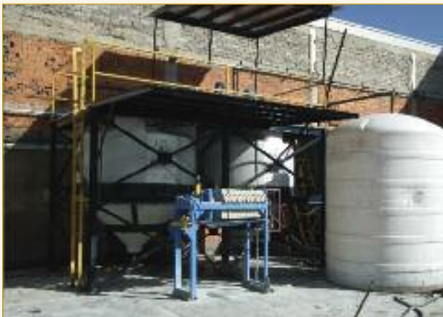
This chrome precipitation plant at Curtec has been recently installed. Out of the 500 tanneries in the cluster, only two have installed these systems to make use of chrome recovery and as part of providing advantage for the CETP.
