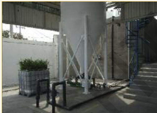
The effluent treatment plant at Lefarc is about to be commissioned. It is intended to provide treated waste waters suitable for washing purposes in the tannery, and for use by the municipality for plant irrigation and washing purposes.
