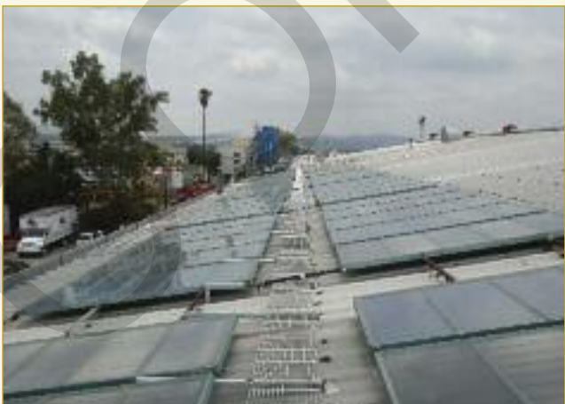
The solar array at Lefarc provides almost all of the hot water to operate the retanning/dyeing department. This hot water can be supported or made up to temperature by direct steam injection if required.
