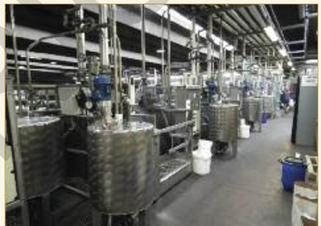
Dani Tannery: The mezzanine serving the retanning/dyeing drums and the experimental dyeing departments are fully fitted with stainless steel. This includes all pipe work, feed hoppers for chemicals, safety guarding and staging.
