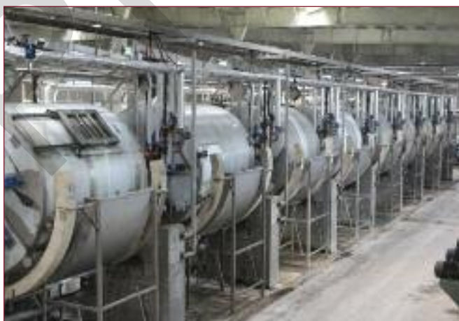
Fully automated Cangilones Next stainless steel drums at Colomer Moda (China).
