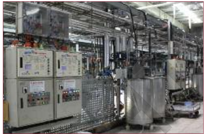
Olcina Automation and Process Control System.
