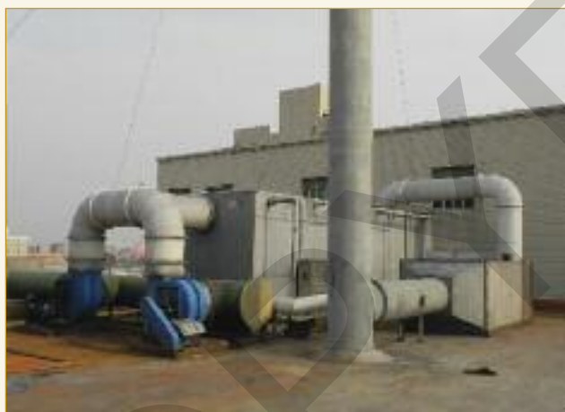
All of the air within the enclosed effluent treatment plant is continuously extracted, then wet scrubbed to remove odour.
