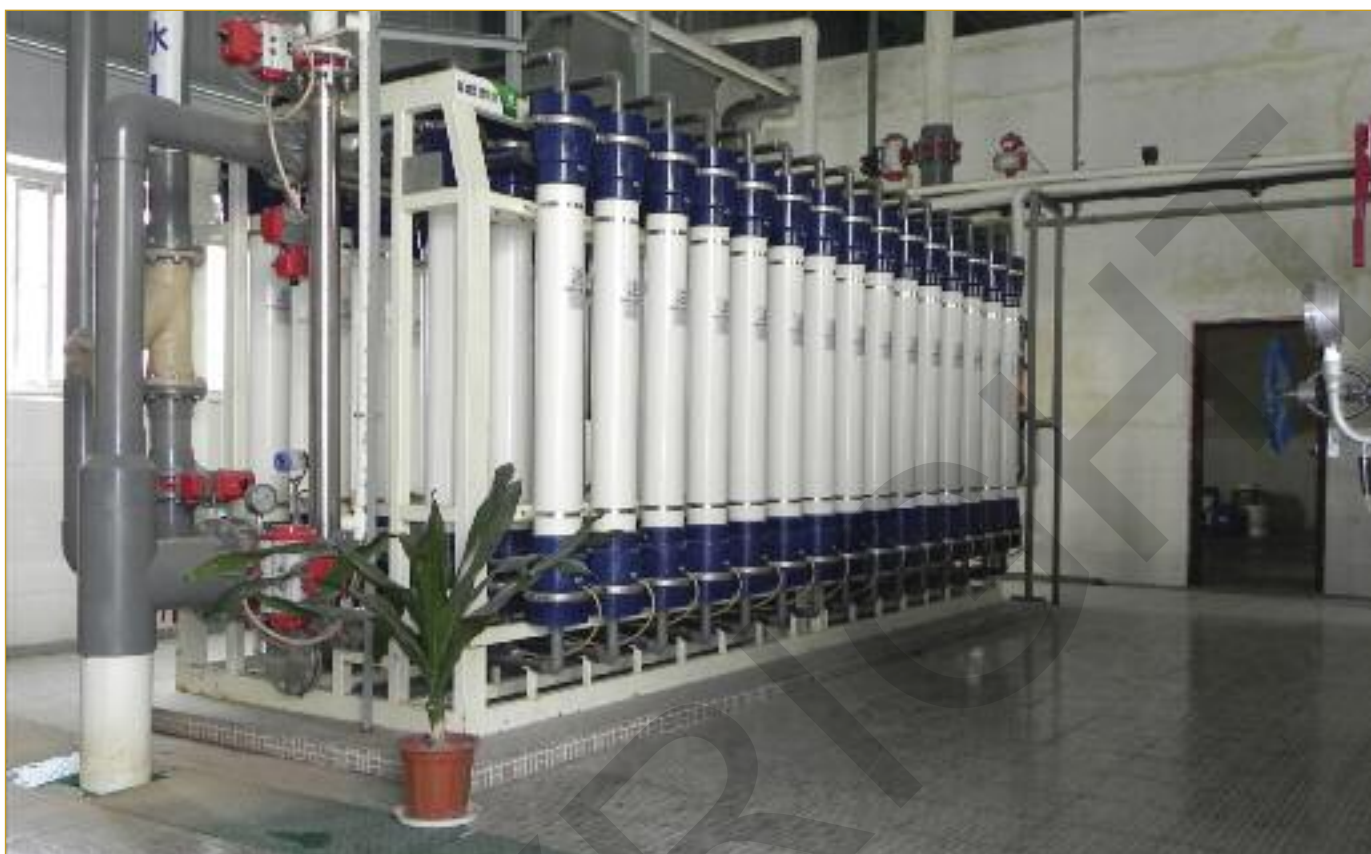
Part of the reverse osmosis plant. Now in operation for one year, approximately 50% of the treated effluent is sufficiently high quality that it is reused in leather making.
