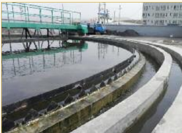
After final settling, the effluent is discharged to the river. This treated effluent is automatically analysed and monitored for COD, N, and chromium.
