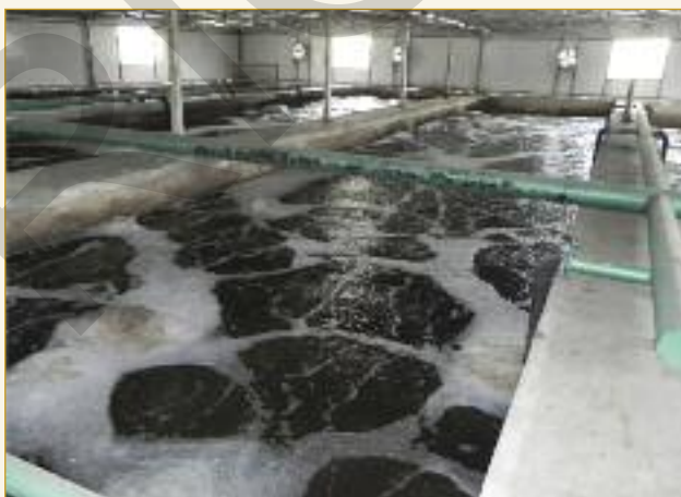
Tertiary treatment comprises a second activated sludge treatment.
