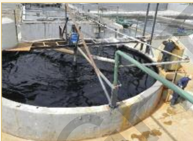
The effluent plant processes up to 3,000 m 3 /day, and the photograph shows the mixing of ferrous sulphate which is used for chemical dosing before the activated sludge treatment.
