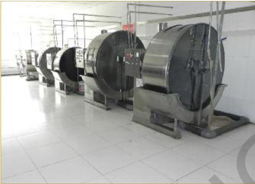
View of the pilot and development plant comprising six drums. In addition there is a set of tumble drums for dye evaluations.
