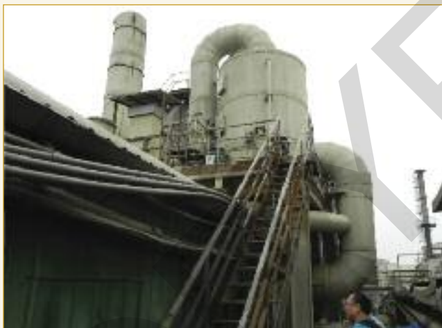
Sulfide oxidation is performed in an enclosed building. A negative pressure is maintained to ensure that odour is fully contained, and the vented air directed via trunking to an air scrubbing unit.
