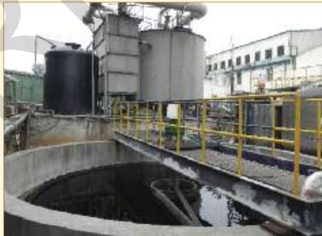
After full biological treatment, the effluent is polished by chemical dosing and settling. Before final discharge from site, the treated effluent is passed through sand filters.
