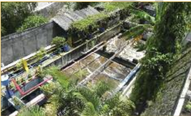
The tannery applies chemical dosing and settling to the effluent before biological treatment. After this treatment the effluent has an extended settling period to remove residual suspended solids, and is then aerated before discharge into the river flowing alongside the tannery.
