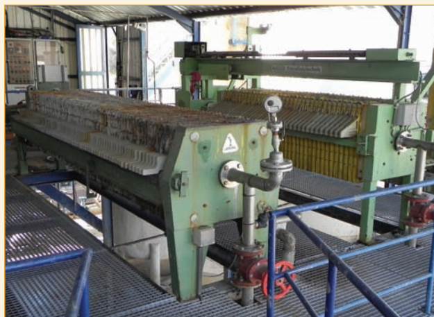
Conventional filter presses elevated to enable easy sludge removal.
