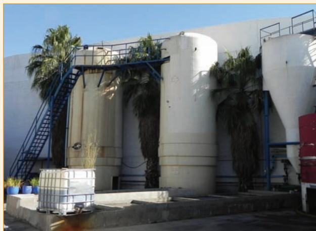
The two aeration tanks were originally used by a brewery, but at 40,000 litres capacity and fully enclosed they are ideal for this purpose.
