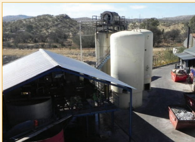
Three inter connected tanks used to mix and balance the effluent flow. A rotary screen is positioned on top of these tanks to remove fine solids.
