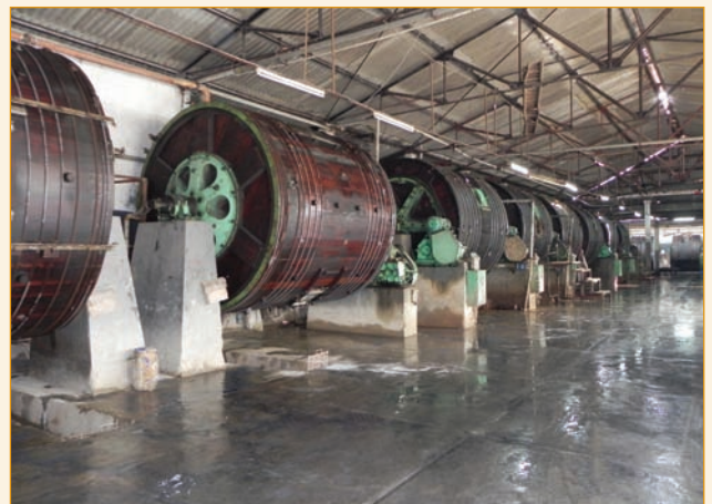
Part of the sheepskin soaking department. After sulfide painting and hair removal by machine, the sheepskins are returned to these drums for liming.
