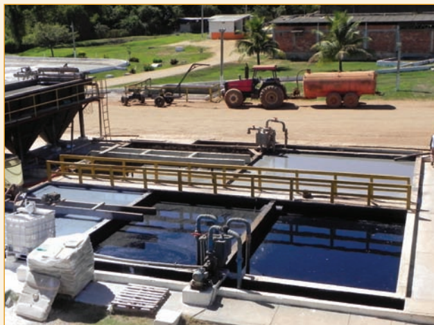
The two sumps used for collection and cooling used chrome liquors and washings are shown in the foreground, with the precipitation sump for surplus chrome to the left. The two sumps for collection of the screened and settled used lime liquors that serve as reservoirs for the recycling system are set behind the chrome recycling plant.
