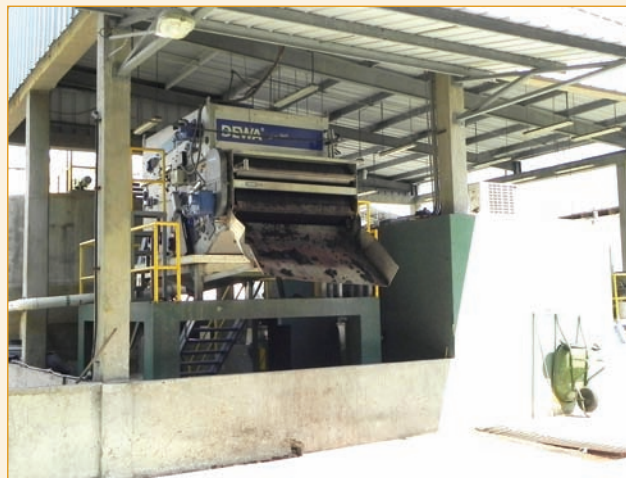
All of the sludges from the effluent treatment plant are dewatered using an elevated belt press.
