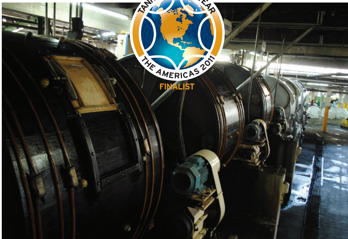
Wooden drums and stainless steel tri-compartmental vessels are installed in the tannery. These suit the processing needs of each different leather type.
