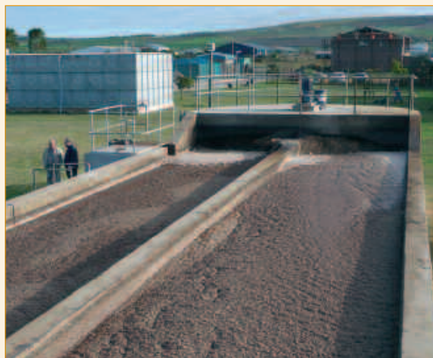
General view of the aeration as part of the activated sludge treatment
