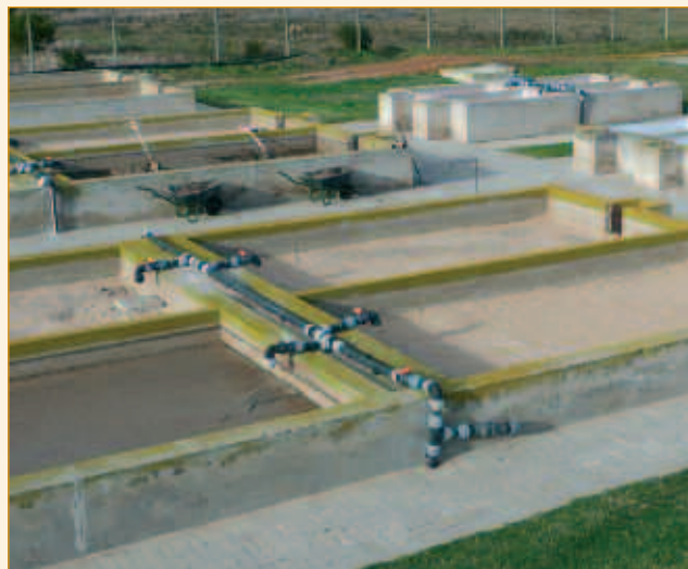
The drying beds for chrome-containing and general sludges.
