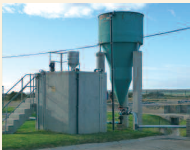
Photo shows the settling tank for chrome precipitates, with the pH adjustment tank to the left.
