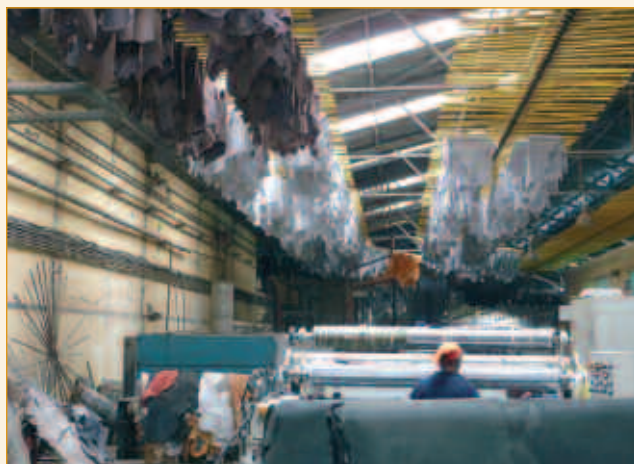
Part of the bovine pole drying conveyor system for side leathers.
