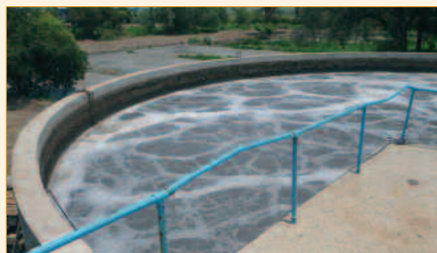
Aeration of raw effluent to equalise and remove sulfides, with sludge drying beds in the background.
