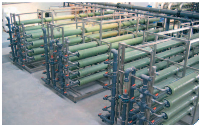
Panel 3: Reverse osmosis membrane plant for high quality water recycling
