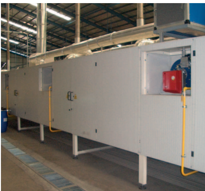
Gas-fired tunnel with burners mounted inside the casing and heat exchange system above (Gemata)
